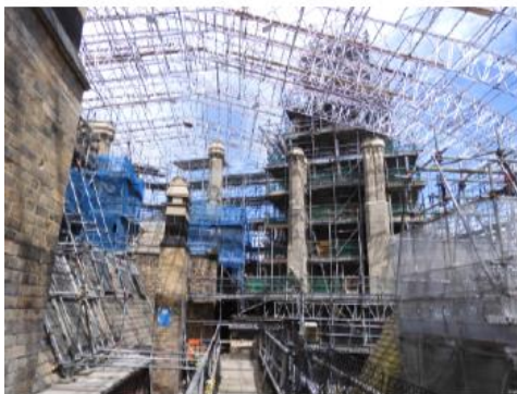
5.111 Chimneys CS34, CS09, CS08 and CS09 on north side of clock tower
