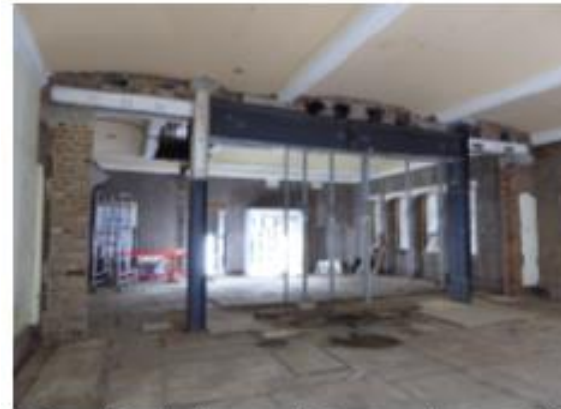
5.15 Removal of needles and props complete from new opening on the east side of room 04-024 Friday 18 March 2022
